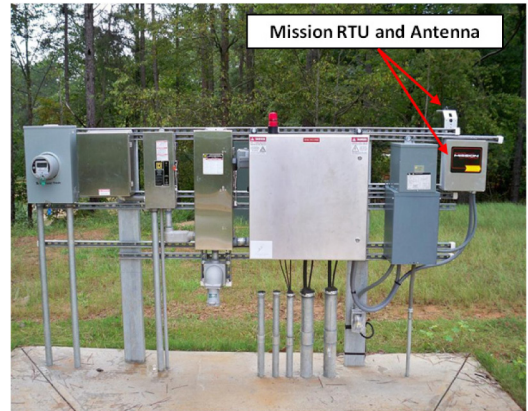
Nema 4 mounted on strut rails
